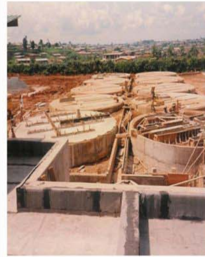
Project: Design/Build Water Treatment Plant – Bumikudu - Nigeria Role: Project Management and Construction Client: FK Construction
