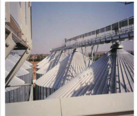
Project: Construction - Eight 25,000 Ton Silos – Ibadan & Jigawa - Nigeria Role: Project Management and Construction Client: FK Construction
